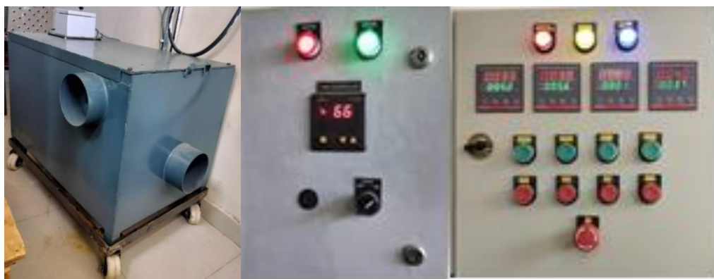
Desiccant dehumidifier with control panel
